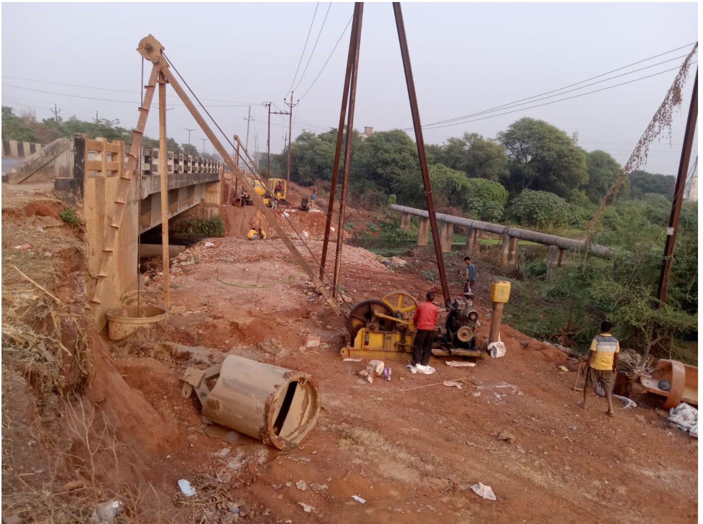
Const. H.L. Bridge at Kosanalla in km 306.00 and construction (Repairing ) of H.L. Bridge at Kharun River in km 283/400 of NH -53.
